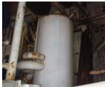
View on Top Part of Existing Mud Gas Separator
