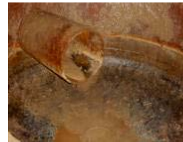
Interior View of of Mud Gas Separator with Pipe Inlet and Bottom Dome End
